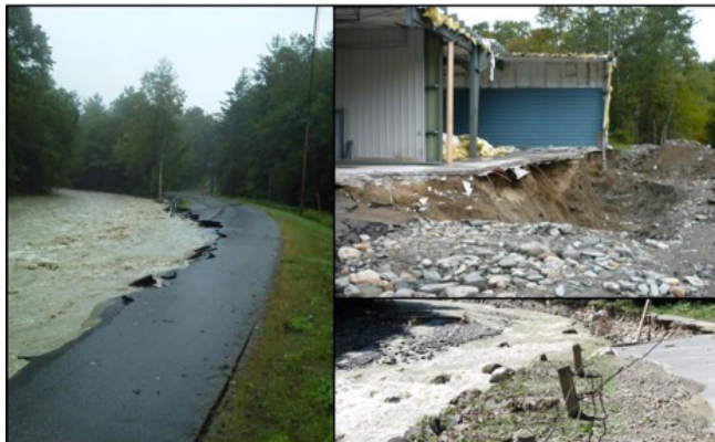
Fig. 2. Flood impacts along the Chickley River during and after Tropical Storm Irene. The picture on the left shows road damage during Tropical Storm Irene. The picture in the upper right shows municipal building damage in Hawley after the storm. The picture in the lower right shows damage along the Chickley River after the storm.
